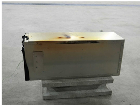
Fig. 14 battery module 10 taken out from the sample rack
